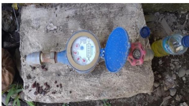
Picture 2. Village PAM Water Network
